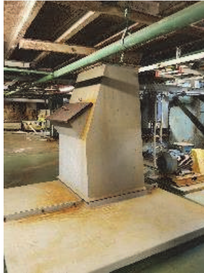
Figure 11. Picture showing the discharge chute for the iron sludge.
